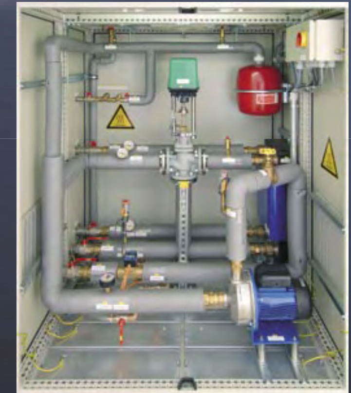
Heat Exchanger Cabinet
